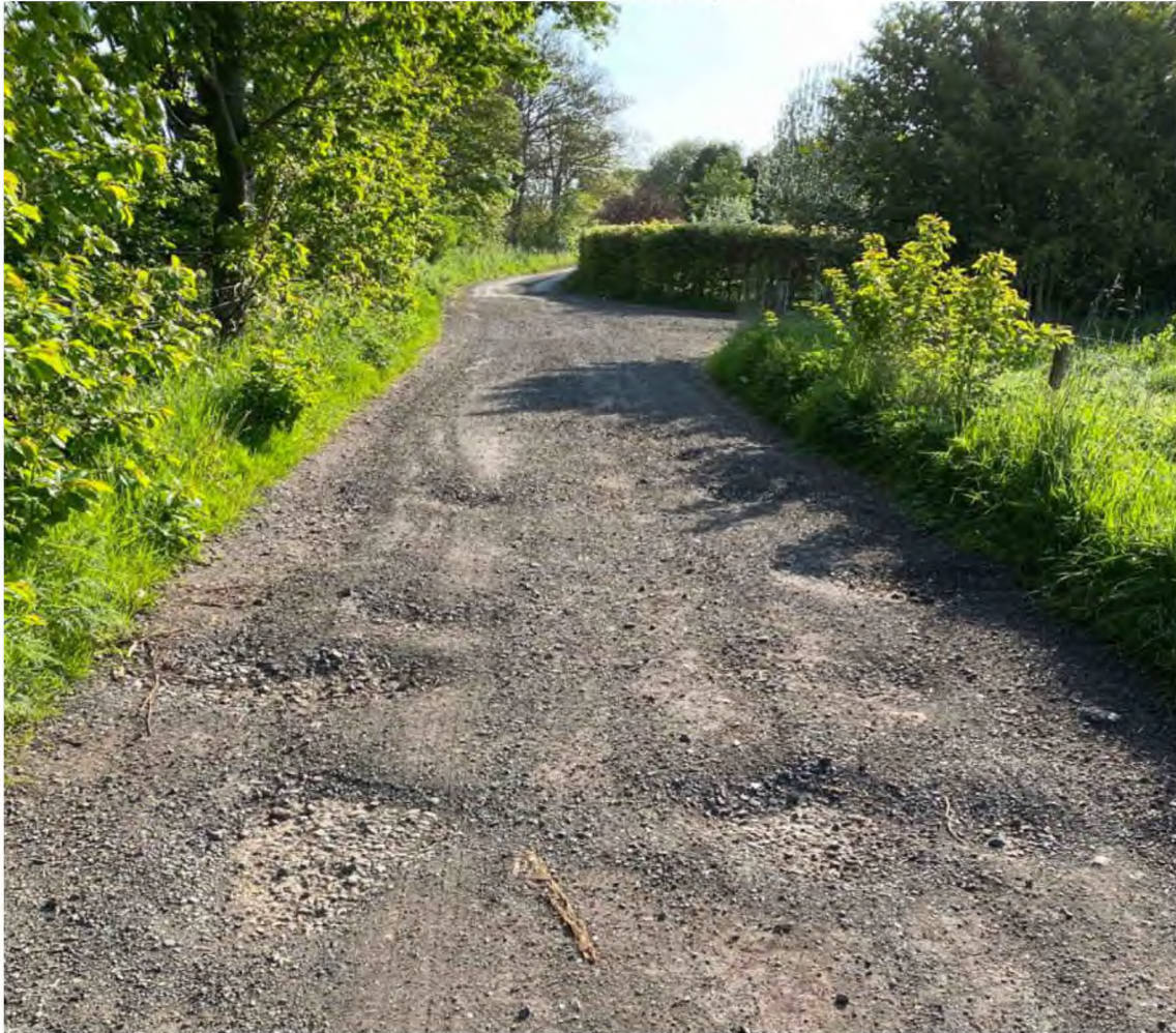
Fig 4: Access track looking East from Highfield, the road all properties use to reach North Lodge, bin collection area and the B6364, dated May 2023
