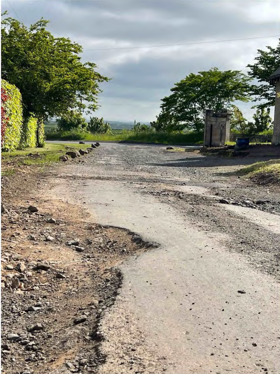
Fig 5: State of the track at the bin collection point at North Lodge, looking East at the B6364, dated May 2023
